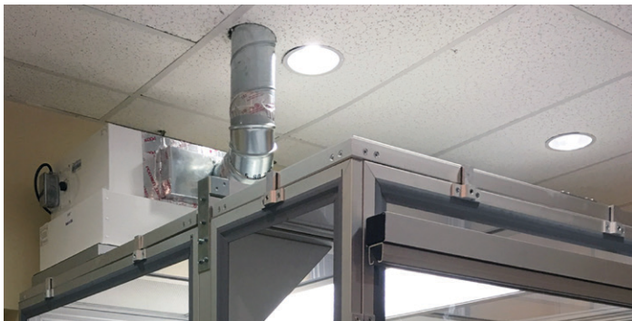
Figure 9: Reverse HEPA fan filter ducted to the building's exterior. This meets USP <800>'s external ventilation requirement.
